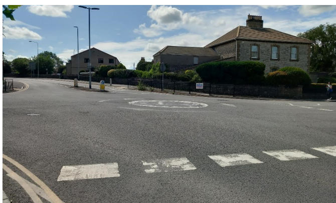
Mini-roundabout—note the worn paint on the central white circle, caused by vehicles driving over it.
